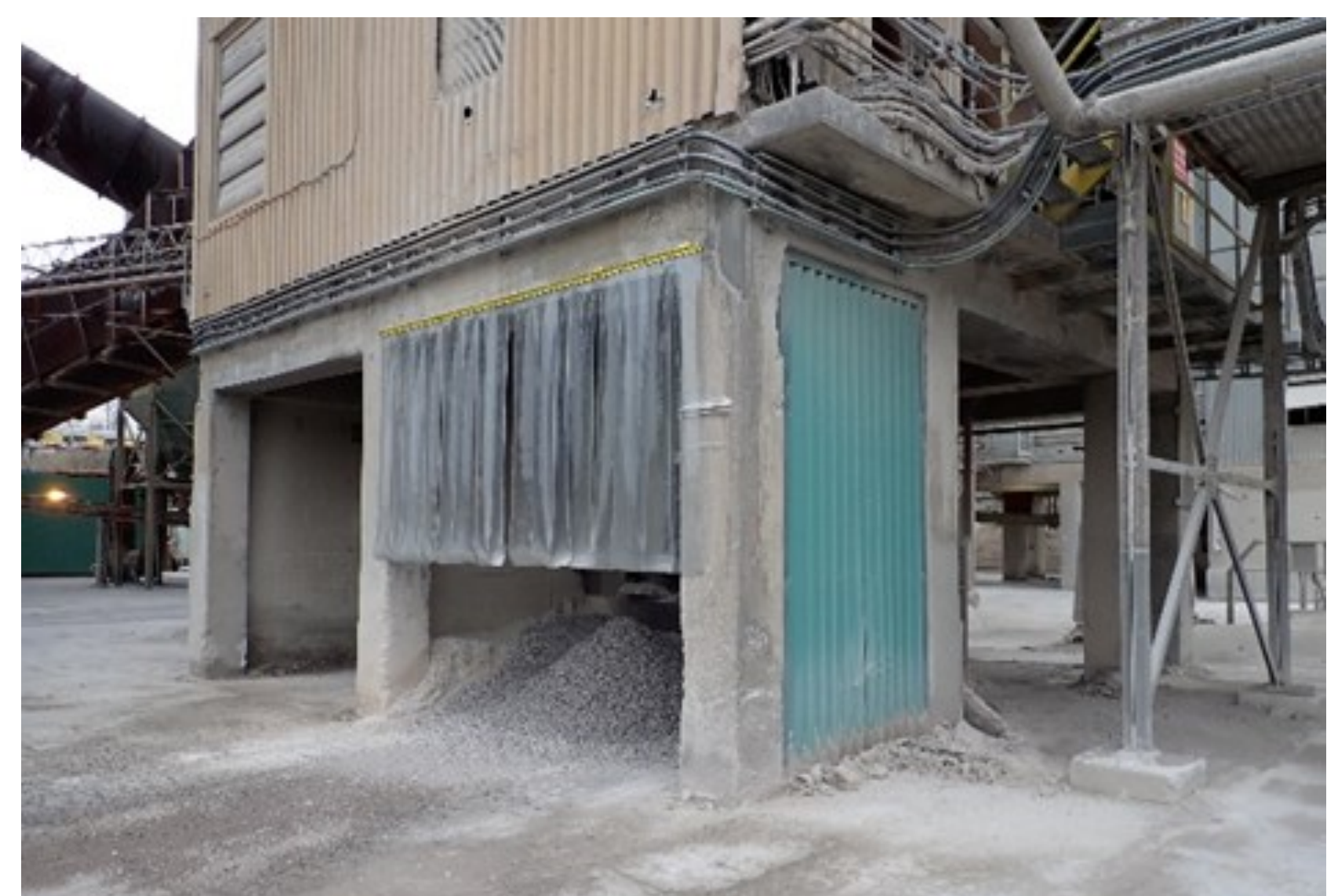
December 2018: Kiln #2 Smoke Chamber Fallout area enclosed with metal sheeting and plastic dust curtain screen
