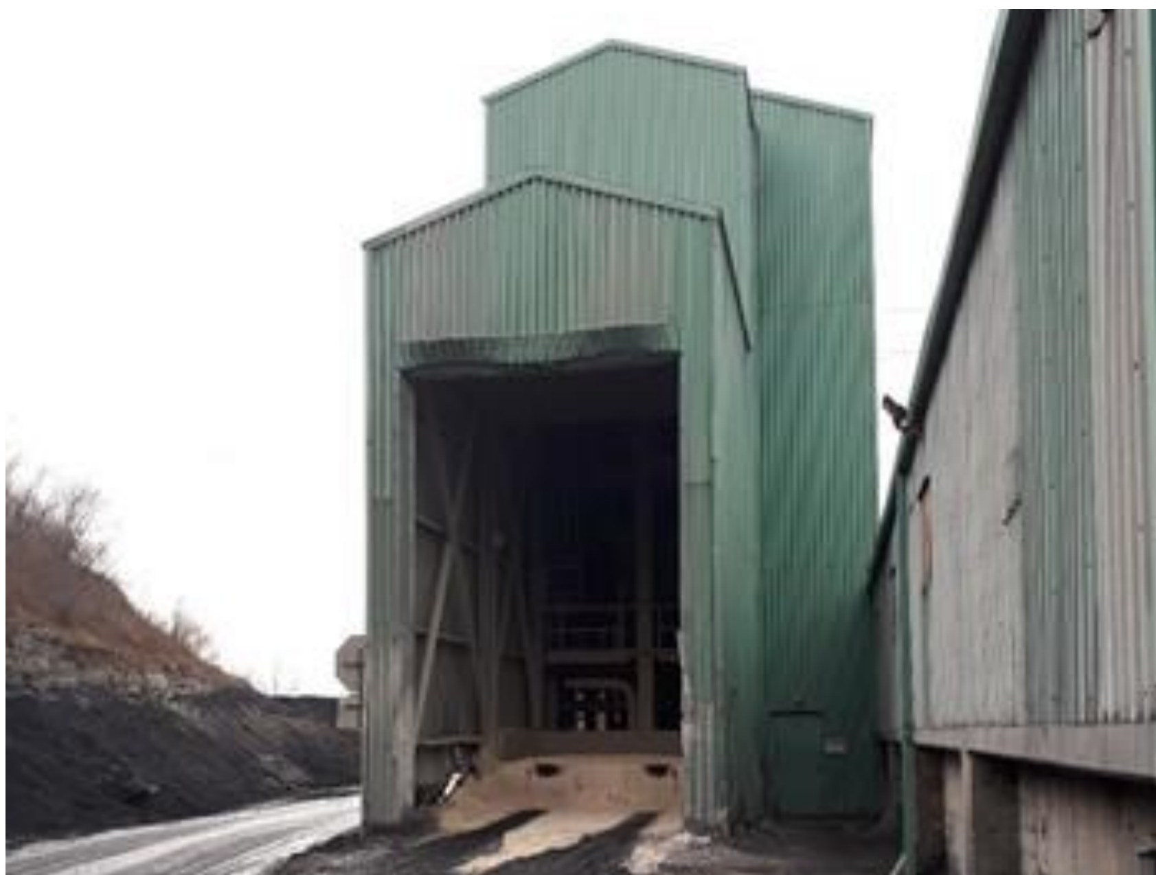
December 2018 Screening Plant Hopper
