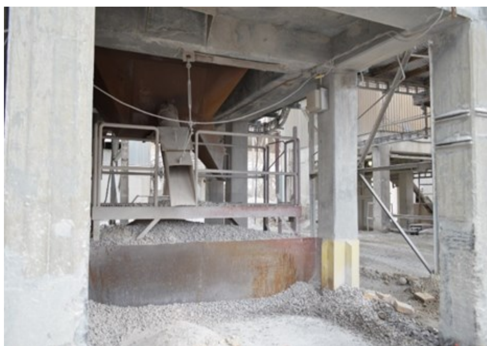
December 2015: Kiln #2 Smoke Chamber Fallout area open
