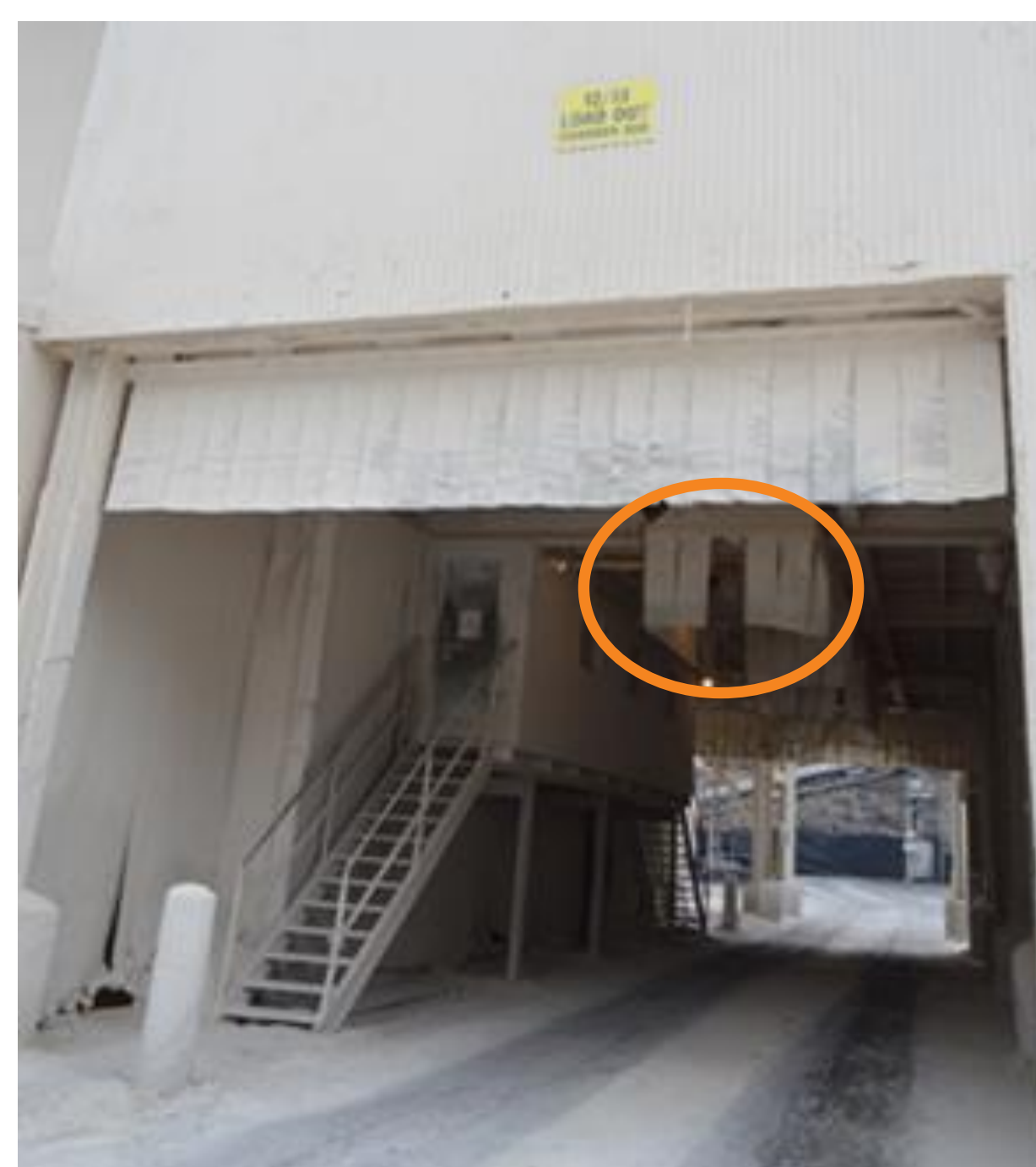
December 2015: Bin 12/13 Loadout with damaged dust curtain (plastic strips)
