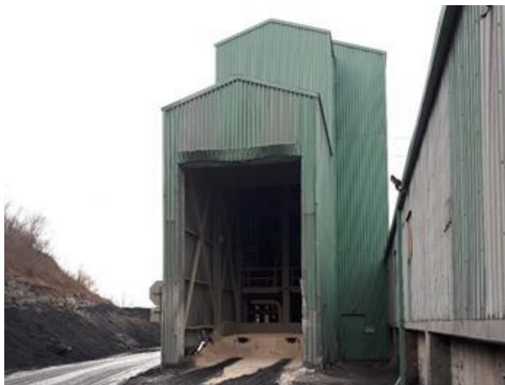
December 2018 Screening Plant Hopper
